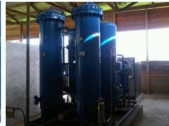
NTK-15P PSA Oxygen Plant - Indonesia
