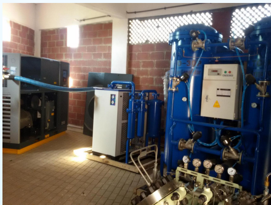
NTK-50P PSA Oxygen Plant - Pakistan Hospital
