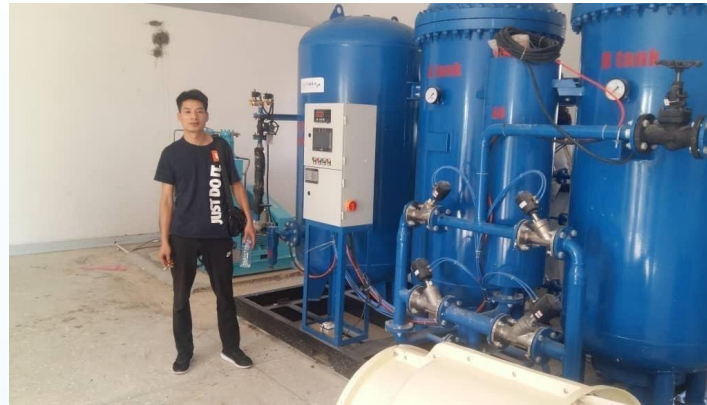
NTK-100P PSA Oxygen Plant - Kazakhstan Hospital
