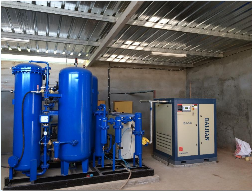
Air Compressor + Oxygen Generator
